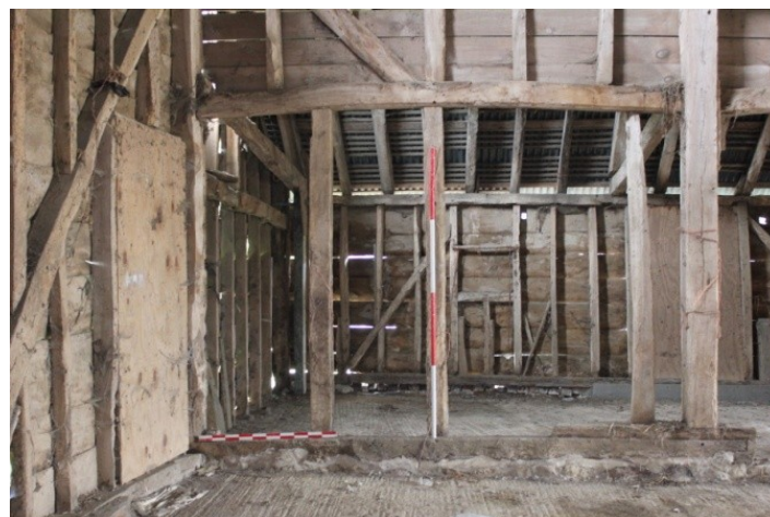
Fig.5. Barn recorded with 1m and 2m scales in the horizontal and vertical plane.
