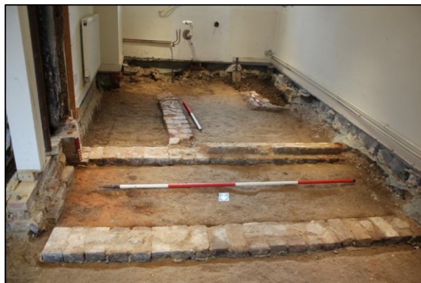
Fig.4. Watching brief undertaken inside a house with exposed features cleaned and recorded before removal.
